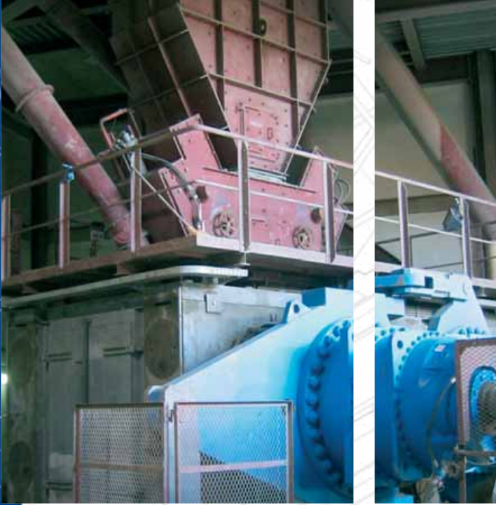
POLYCOM® for clinker grinding in a combi grinding system in the Lebanon.
