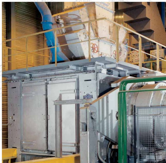
POLYCOM® for cement finish grinding in Belgium.
