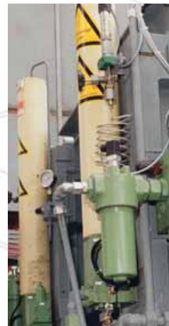
The hydraulic system includes the pressure application and spring systems with pressure cylinders and piston accumulators.
