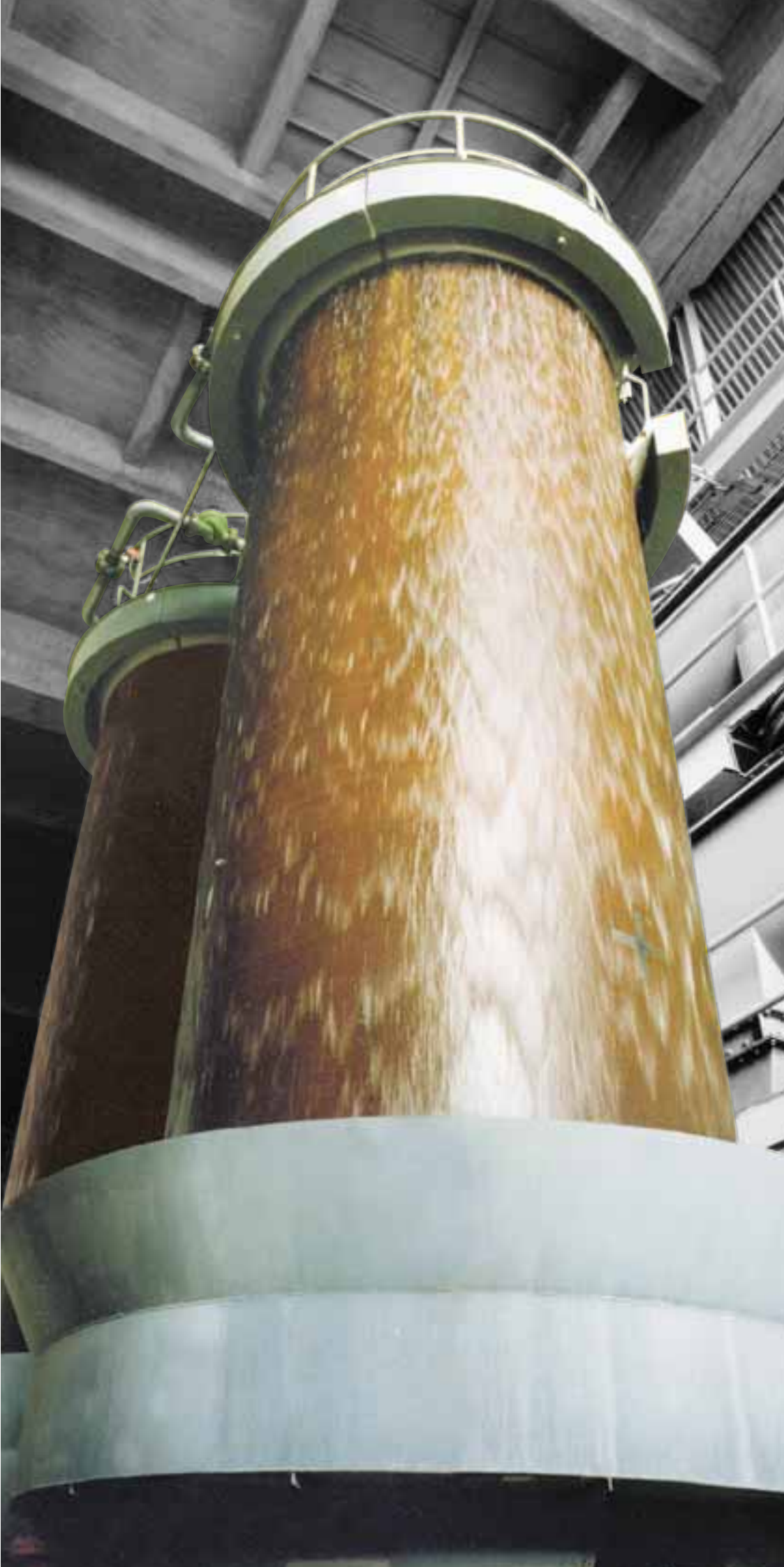
Two fines coolers in a cement grinding plant.
