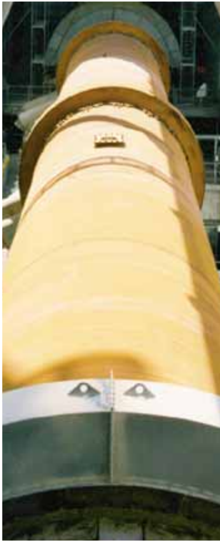
5,000 tpd cement clinker kiln on 3 roller stations.
